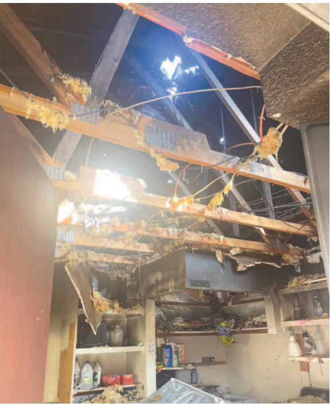
Fire gutted the Outrigger Motel in Grove Friday night.
