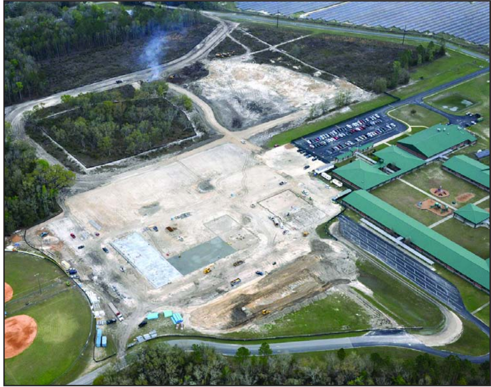
Construction is underway at the site of the new Perry Primary School. In a move to cut costs, a decision was made to move the site closer to the existing Taylor County Elementary School. A retention pond will also be added, shown at the top right.
