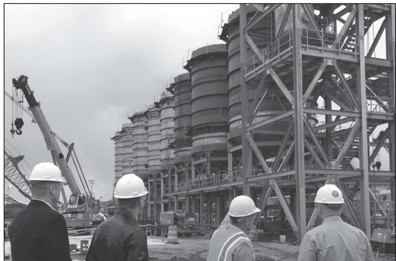
A delegation from the Florida Department of Environmental Protection (FDEP) observes construction progress of the Black Liquor Evaporator (BLE) project during a tour of the local Foley Cellulose mill provided by Fenholloway Project Leader Chet Thompson. Shown above are: (l to r) Greg Strong (FDEP), Jim Maher (FDEP), Thompson and FDEP Secretary Noah Valenstein.
