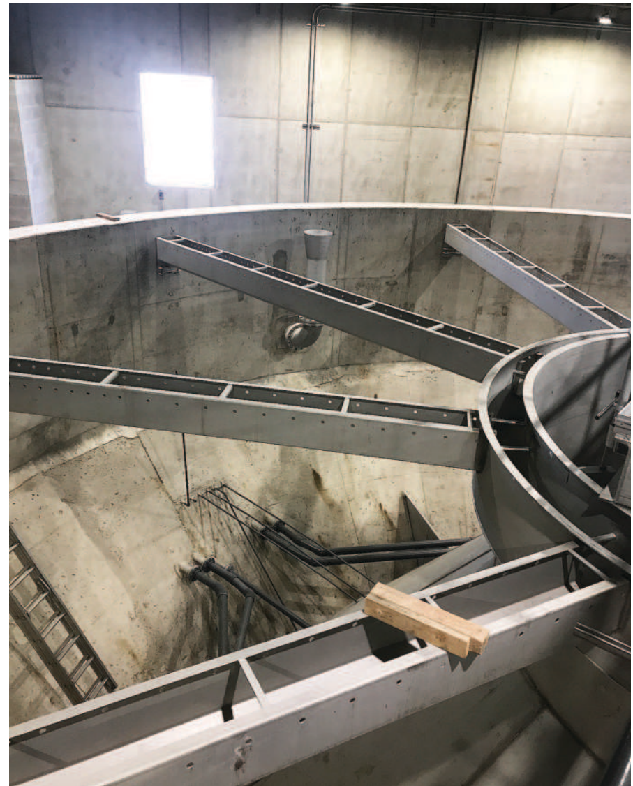
Shown above is one of two new solid contact units at the water treatment plant. When in operation, the basin will be full of water.
