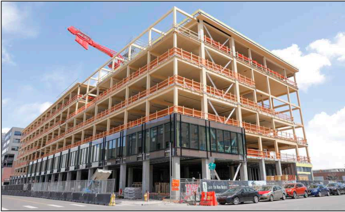
Timber project T3 RiNo was topped out and will be completed later this year.
