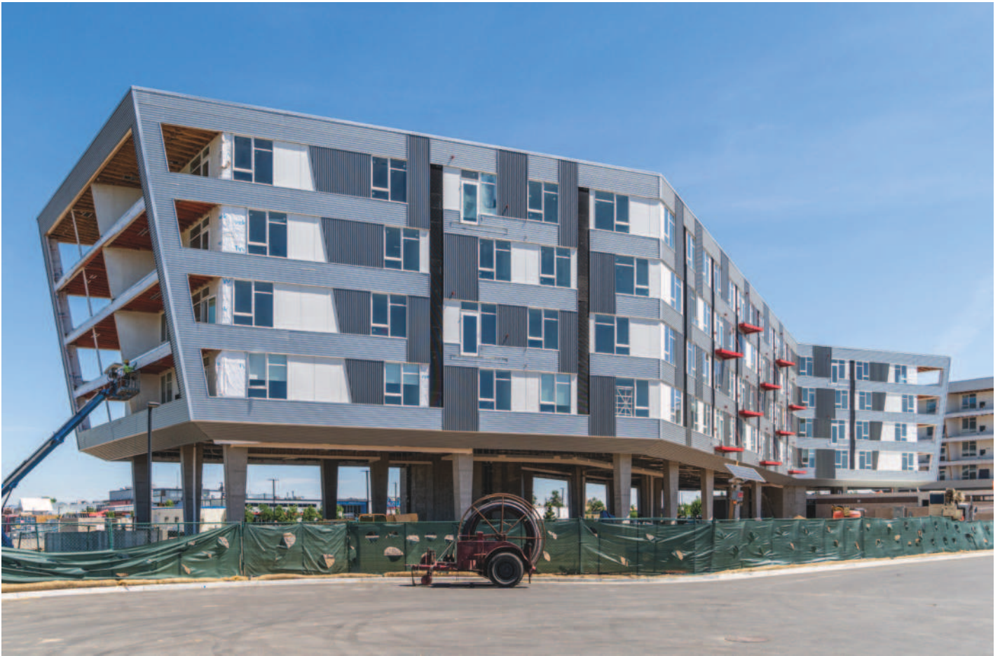
The new Stanley House speaks to Stanley Marketplace architecturally as well as operationally.
