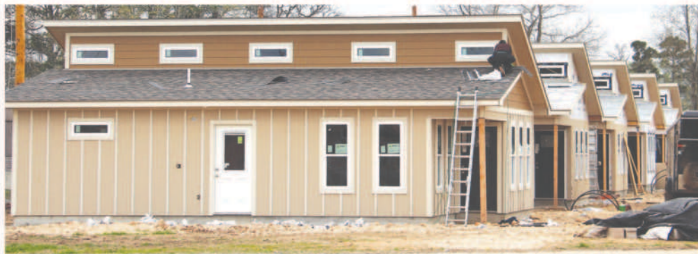
Two bedroom rentals for 55 and over being constructed at Highway 59 and 20 in north Jay.
