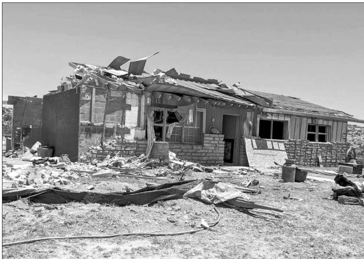
This is a photo of former Alpine Buck Christopher Matthew Galvan's grandmother's house after the tornado blew through Sanderson this past Sunday. Galvan along with many others in Sanderson need donations in the form of household goods and other items that were completely lost in the storm.
