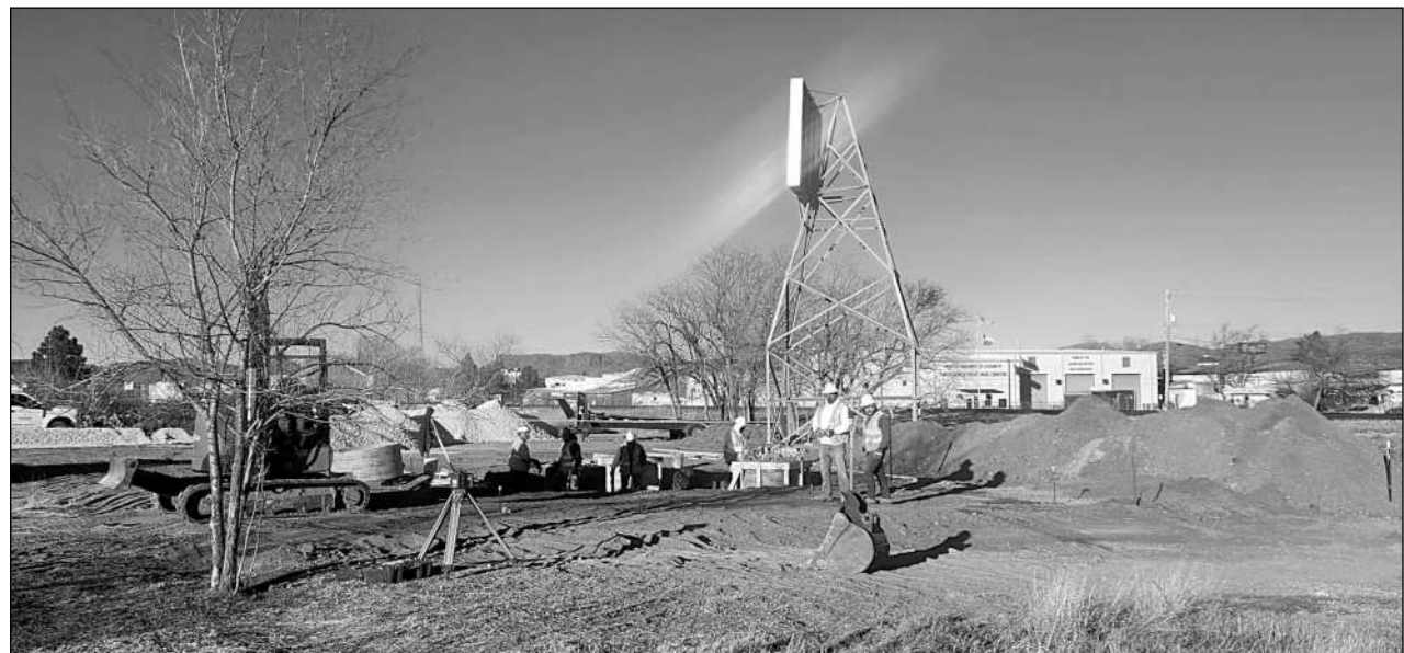
Construction crews work on building a new tower on Murphy Street for the Union Pacific Railroad.
