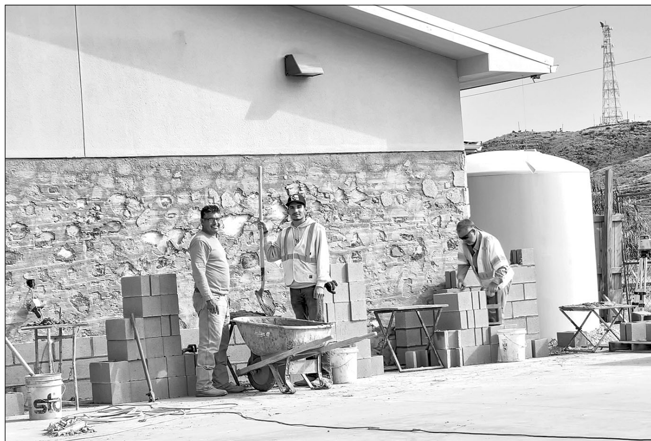
Construction workers are making progress on the Alpine Public Library remodel. After the demolition of the old awning and porch, a new slab was poured and completed just prior to the holidays. Construction on the firewall required for the build is now underway.
