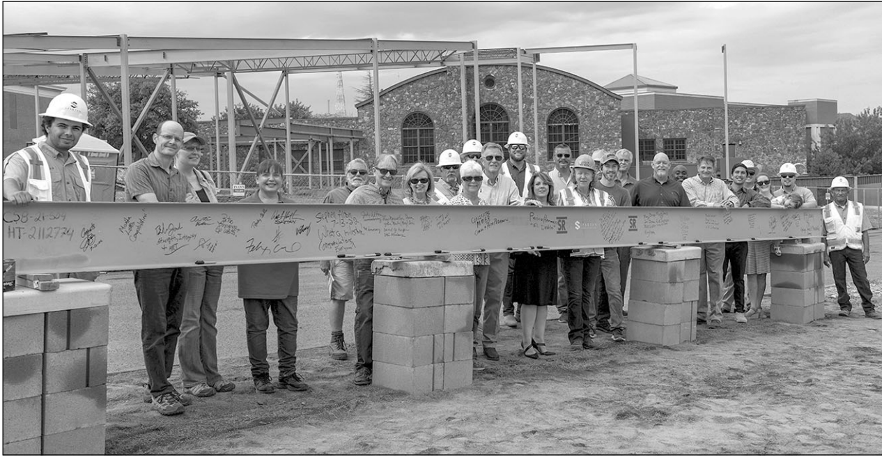
Museum of the Big Bend at Sul Ross State University hosted a group to “Sign the Beam” on July 13. The topping out event celebrated a milestone in the construction of the museum’s new wing - the beam’s placement at the building’s highest structural point. Those in attendance were invited to sign their names, and add well wishes for success and for safety of the crew.
