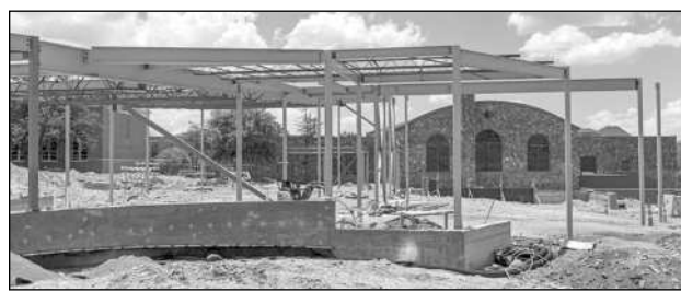
Construction on the Emmett and Miriam McCoy building is expected to be completed in early 2023.
