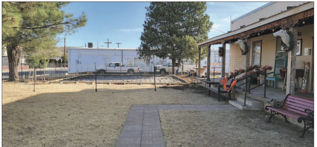
Construction of additions to the Alpine Visitors Center is underway, including a new pavilion.
