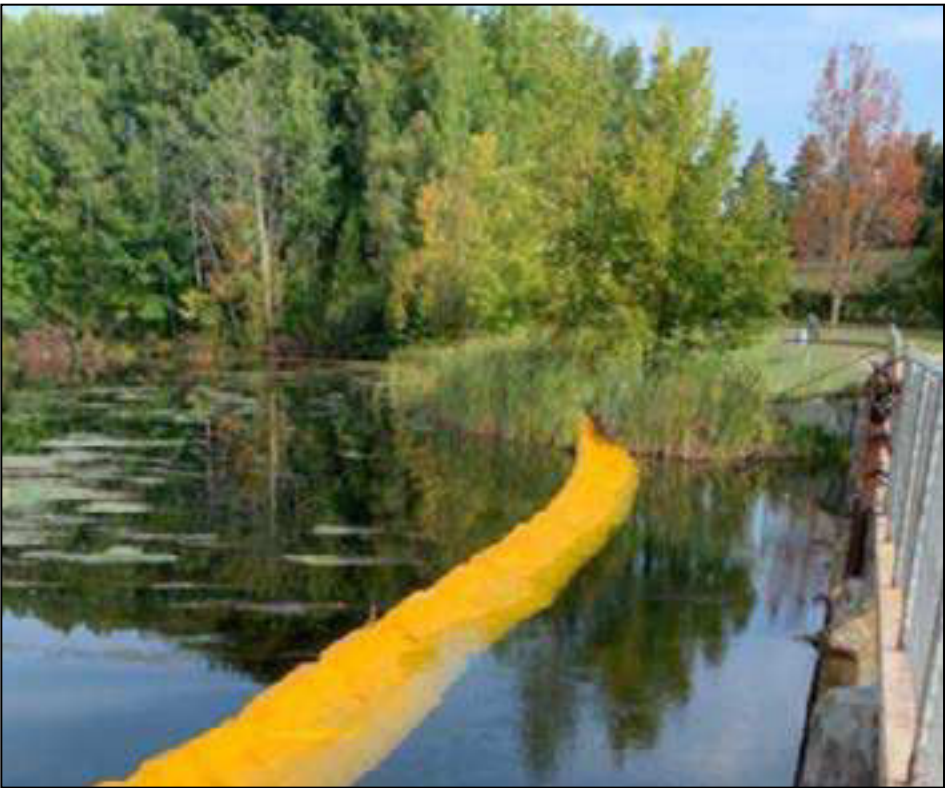
Turbidity curtains will protect the dam at Shamrock Lake while the lake is being dredged.
