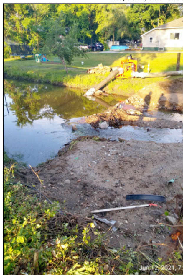
Heavy rain caused flooding which damaged the site of the sixth street bridge project Photo courtesy of Drain Commissioner Carl Parks
