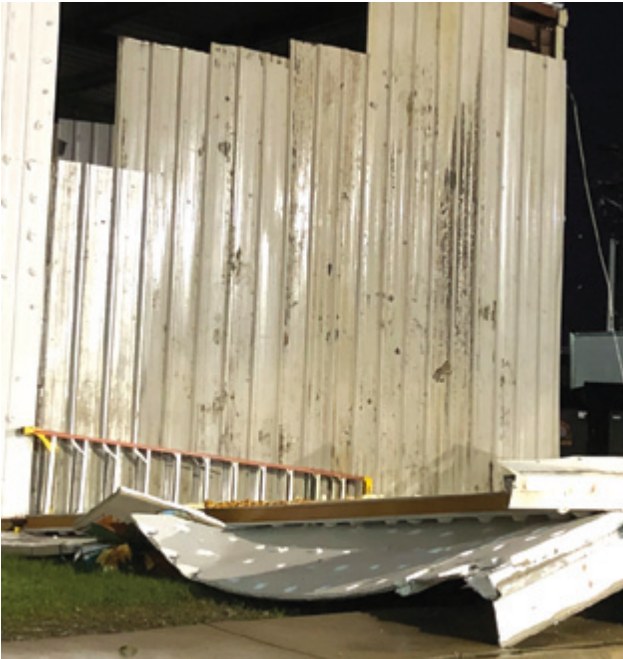
A WALL COLLAPSED AT SLOVACEK'S during last Wednesday's storms. Large hail and winds up to 80 mph caused damage throughout the county. -- Tribune photo by Denise Hornaday
