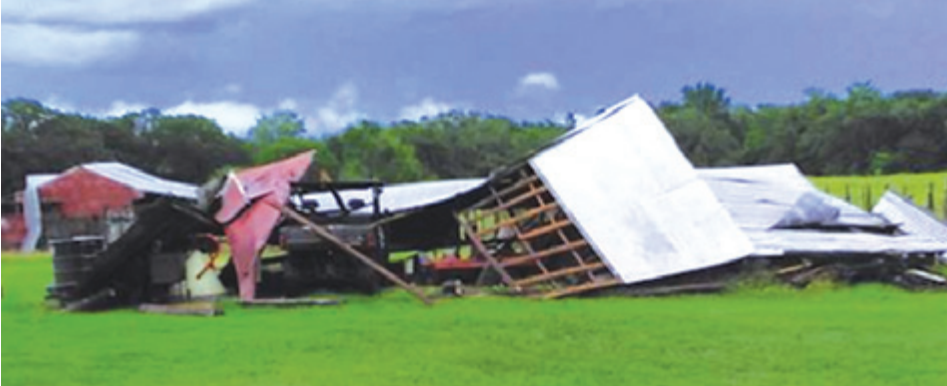
DAVID MCMAHAN LOST THIS STRUCTURE during last Wednesday's storms due to high winds. This picture was taken between Caldwell and Tunis on F.M. 166 in Burleson County.
