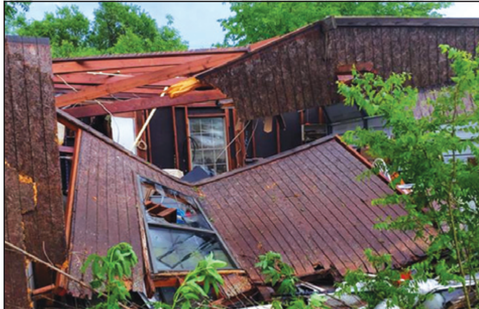
THIS BUILDING ON DAVID STONE'S property off County Road 272 suffered extensive damage due to the thunderstorms last Wednesday. High winds gusting up to 80 mph, large hail and a possible tornado damaged many buildings and crops throughout the county.
