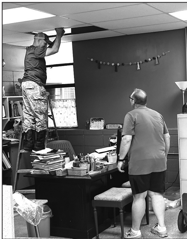
Several improvement projects were completed at Good Pine Middle School as part of the LaSalle School Serve Day September 16, including the installation of ceiling tile in several classrooms.
