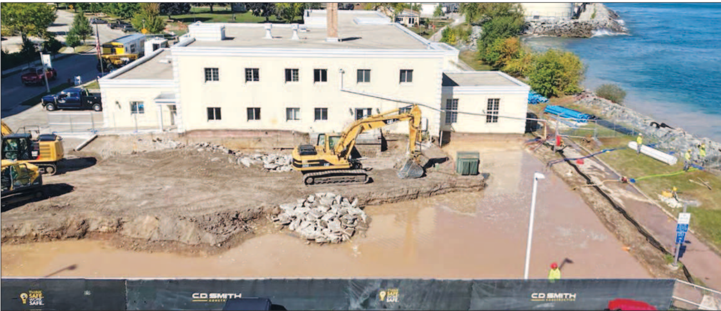
AFTER A WATER MAIN broke while crews were excavating just south of the Port Washington water plant at about 1 p.m. Friday, contractors pumped the water off the site and into the lake to help facilitate repairs.
