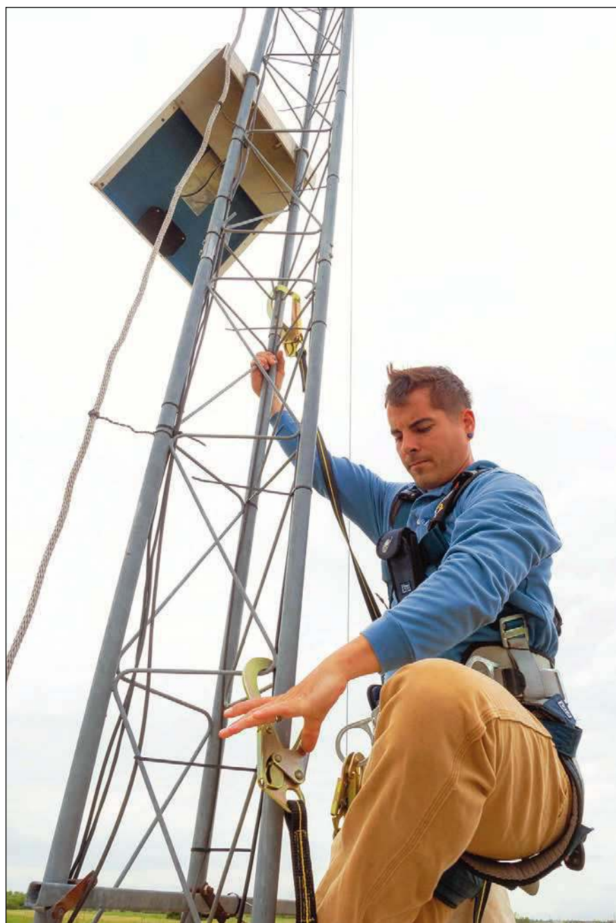
Mesonet field technician Aaron Beckwith is climbing, in a safety harness, to reach the top of the 10-meter Mesonet tower. Wind and air temperature sensors are located at the top. The technician must climb the tower to replace these instruments or perform repairs. Seen just above his head is the back of the solar panel which powers most of the instruments on the tower. (Photo provided)
