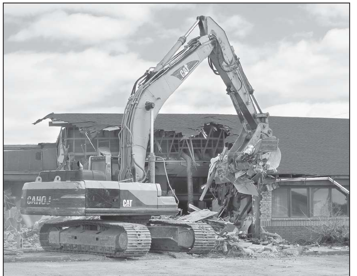
A Colby landmark, the Sirloin Stockade building on South Range Avenue that became Montana Mike's, fell to a wrecking crew (below) as the land was cleared for the construction of a new Casey's General Store. Work would later stop for several weeks as the virus pandemic halted many projects. EVAN BARNUM/Colby Free Press
