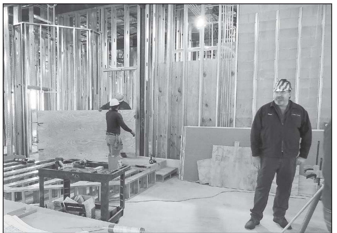
Work on the Thomas County Justice Center continued (above), with interior metal studs going up where the walls would be. The City Council toured the building, stopping in one of the two courtrooms, where workers shaped plywood on the elevated platform where the judge would sit.
