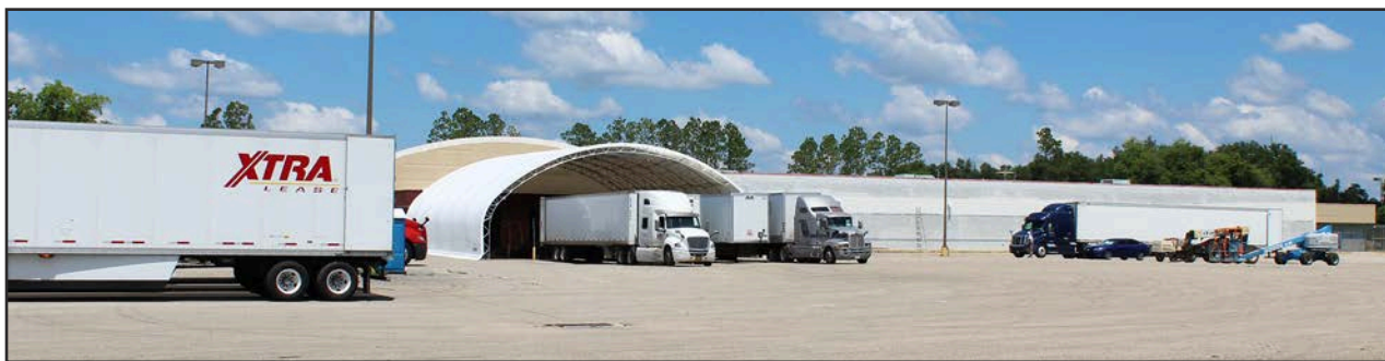
New construction is ongoing at the Super-Pufft South Warehouse (former Kmart building) location, where eight new shipping docks are currently being installed on the south side of the building to allow for a more efficient shipping and logistics system.
