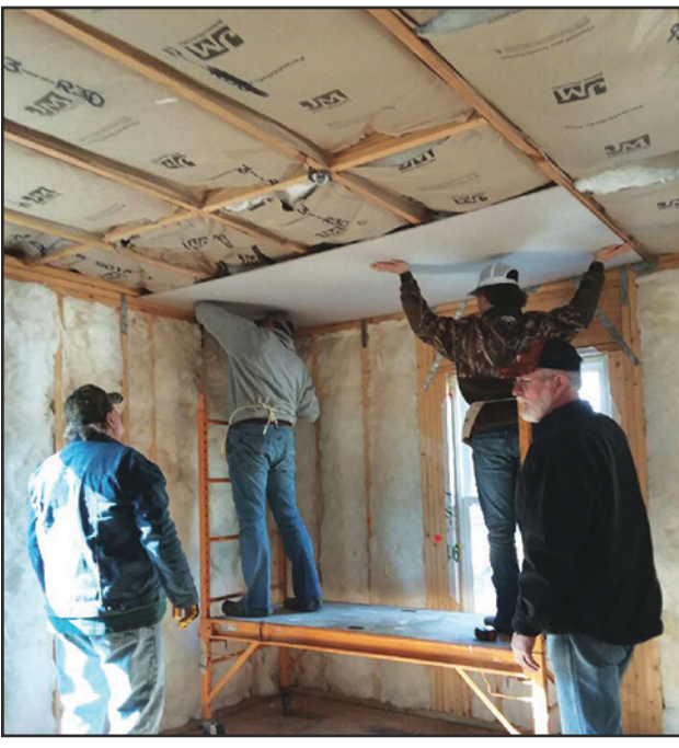
Volunteers are needed to help with finishing drywall, installing cabinets and painting.
